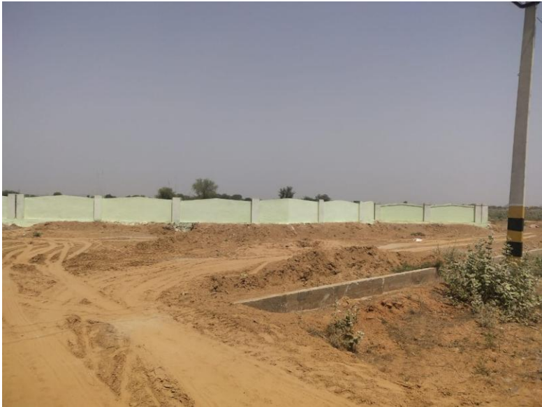
Construction of road & CD works in newly planned area at Ind. Area Ghiloth
